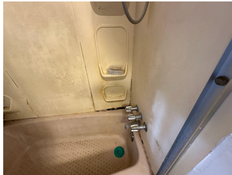
Mold in Bathroom
